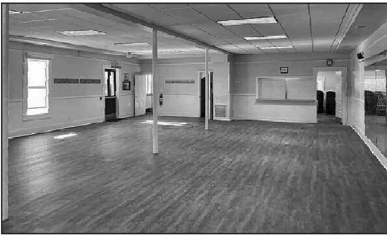
Left Hand Grange has new luxury vinyl flooring on the first floor.
